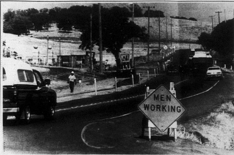
Residents traveling on East Natoma heading out of town toward El Dorado Hills have noticed a lot of construction activity near Folsom Prison. The road work will consist of a widened road
